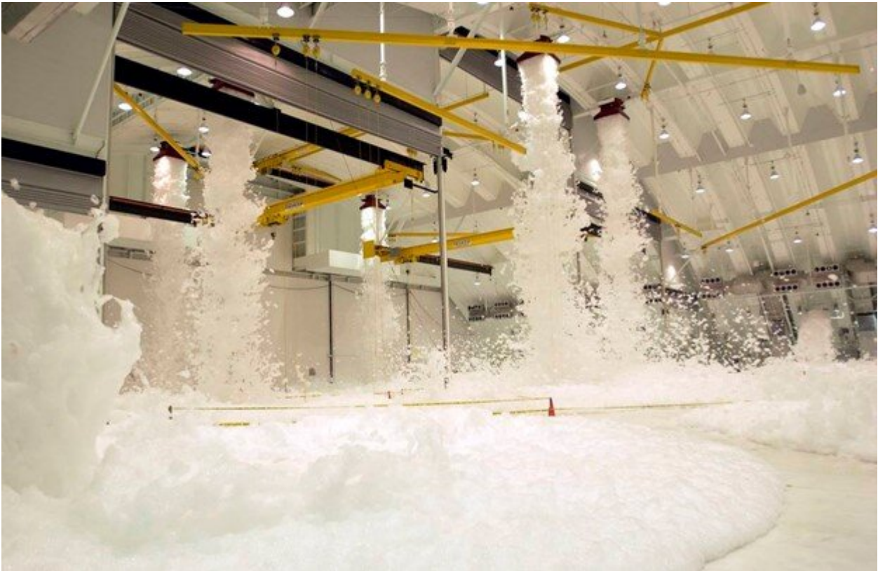
ANDERSEN AIR FORCE BASE, Guam — Foam from a fire suppression system sprays from the walls and ceiling inside a newly built aircraft maintenance hangar during a test and evaluation exercise in 2015. (U.S. Air Force photo)
