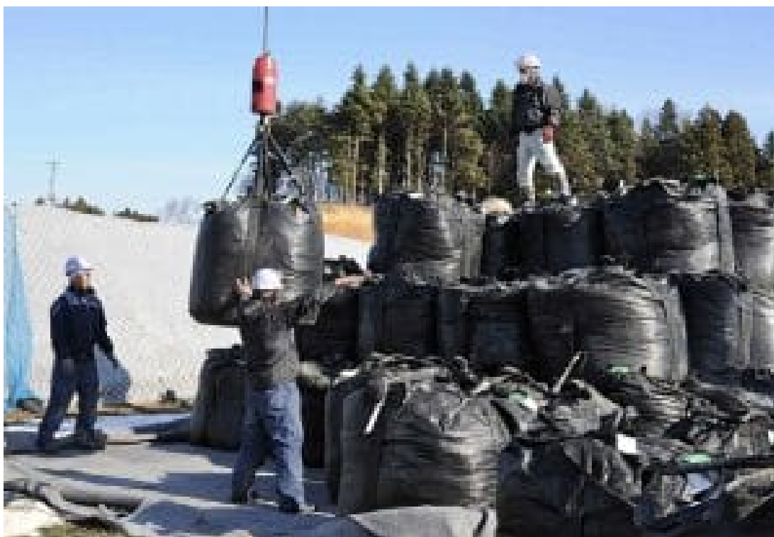
File photo of workers stacking bags of soil collected during Fukushima’s so-called decontamination and cleanup operations, a few months after the accident. Image courtesy of Ricardo Herrgott/Global 2000.
